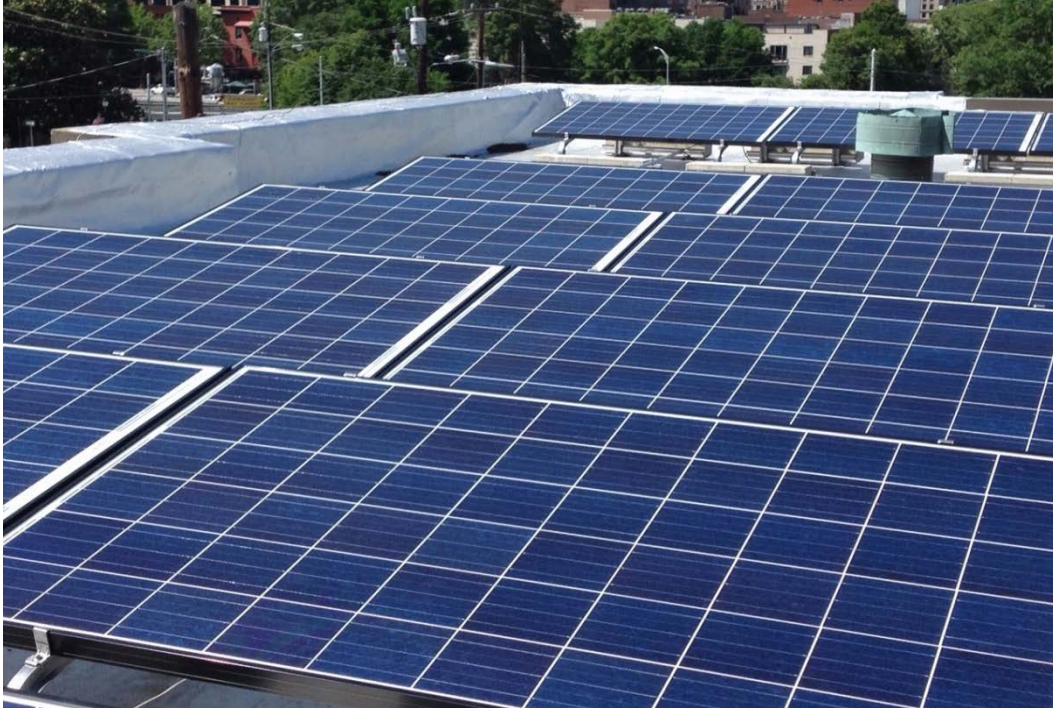
5 kW solar photovoltaic installed on the rooftop of Faith Community Church, 417 Arlington Street, Greensboro, NC 27406
