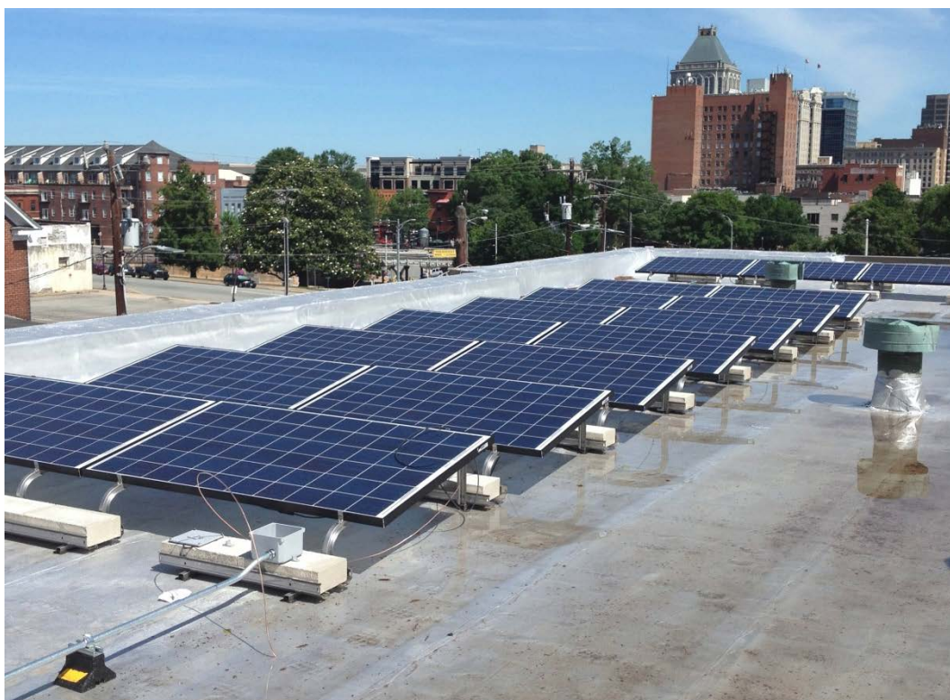
5 kW solar photovoltaic installed on the rooftop of Faith Community Church, 417 Arlington Street, Greensboro, NC 27406
