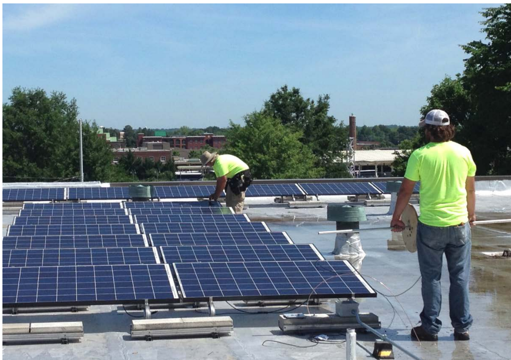
Installation of 5 kW solar photovoltaic system in progress on the rooftop of Faith Community Church, 417 Arlington Street, Greensboro, NC 27406
